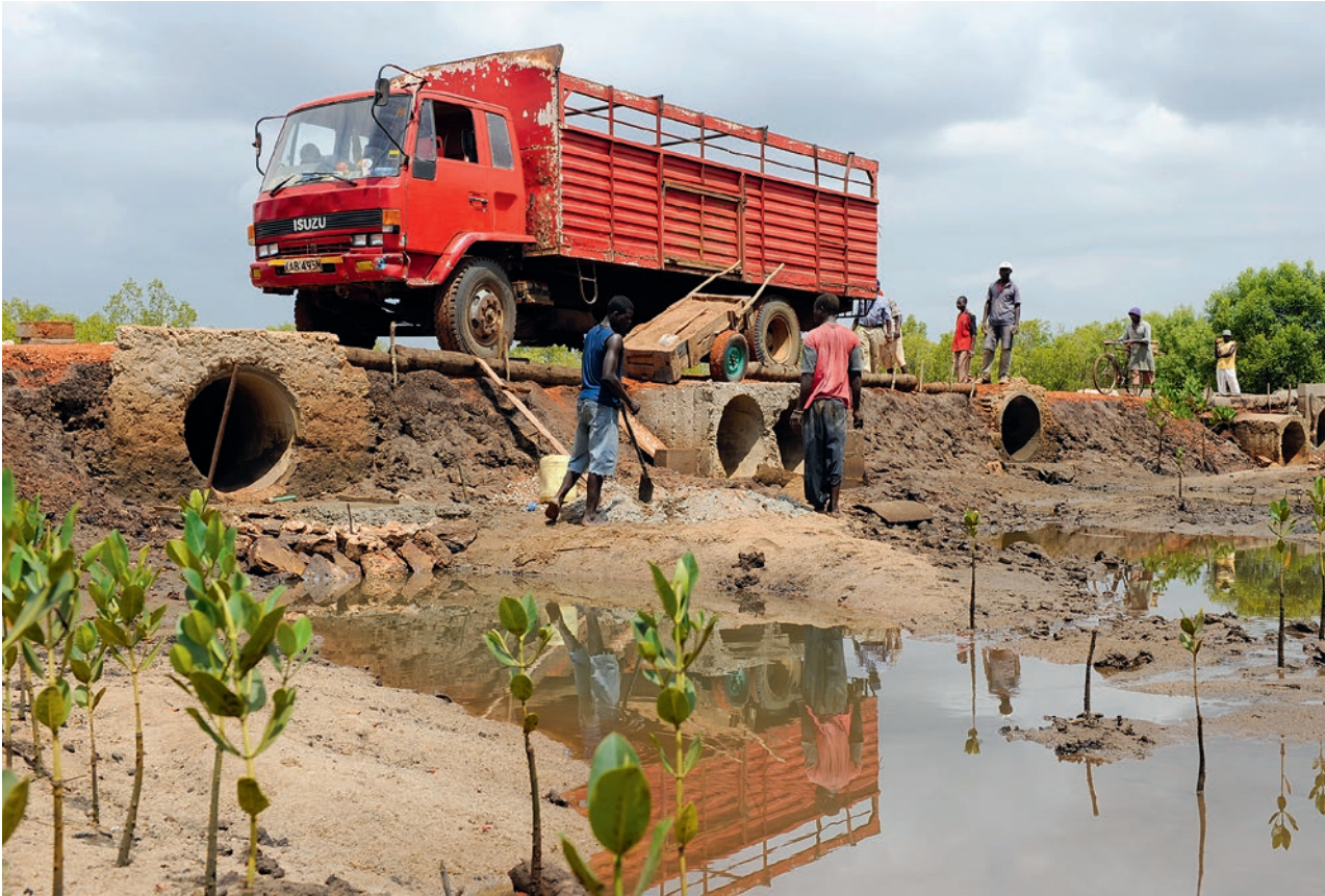
Well-run development banks can ensure long-term finance for key development sectors and sustainable infrastructure like building roads to connect small and remote villages and enable their market access. Here the construction of a road between villages near Mombasa in Kenya.
